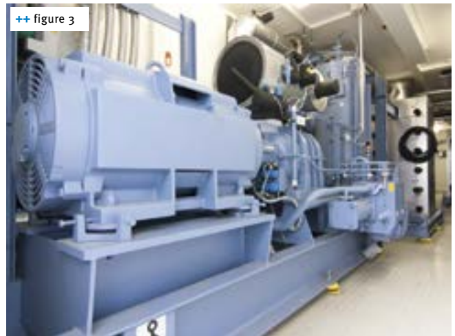
++ figure 3 GEA Grasso chiller in spacious container
