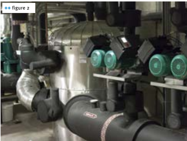
++ figure 2 Temper brine valves in the central machine room
