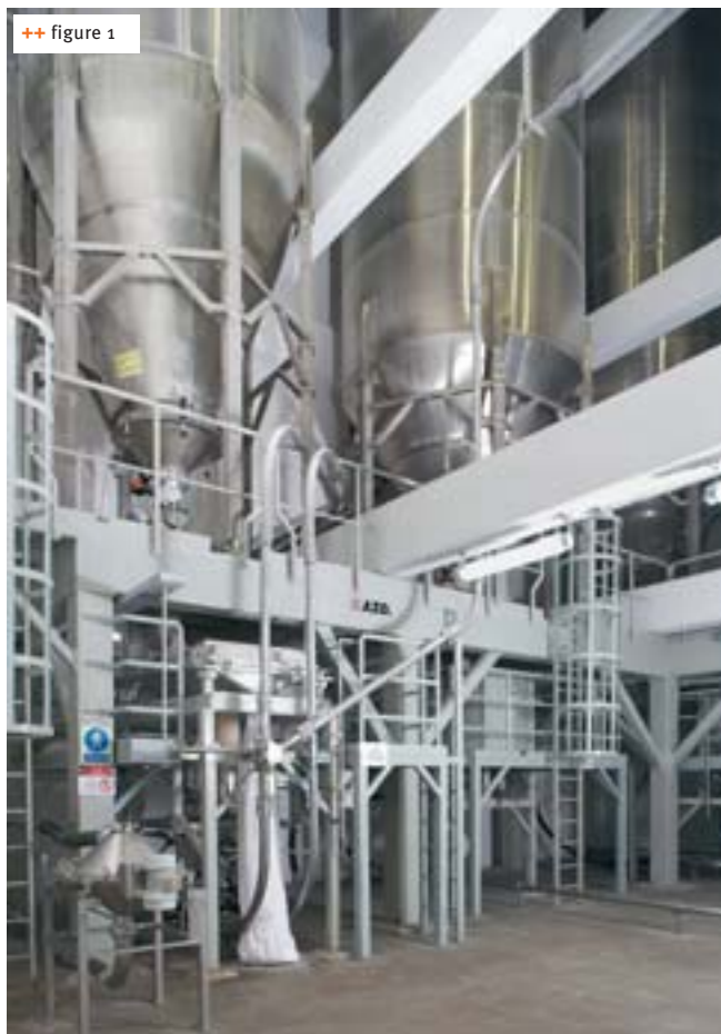
++ figure 1 Indoor silo for flour (left), indoor silo for sugar (right)
